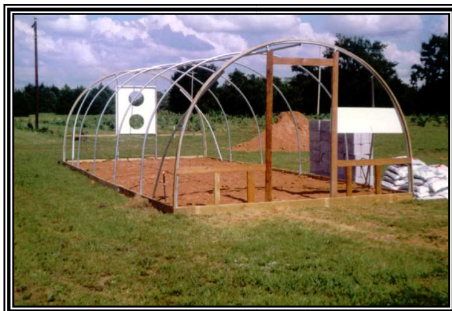
This is such a good example of GH construction I had to add it again. Note also the earth grade work inside the frame work. Slightly raised above outside grade.
